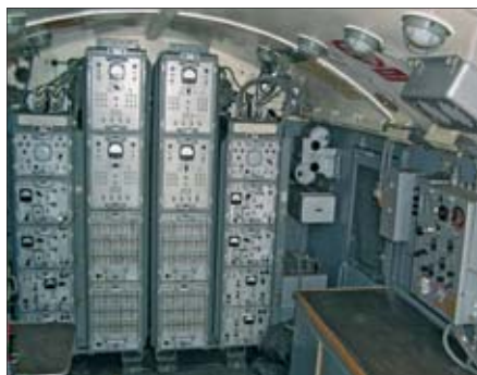
R 404 radio-relay station
